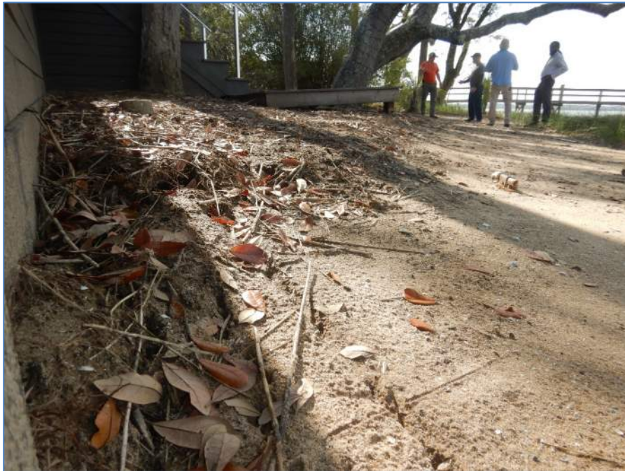
Photograph 12: Meeting with KICA and Town Personnel, Eroded Scarp in Foreground, Unlevel Landing in Background
