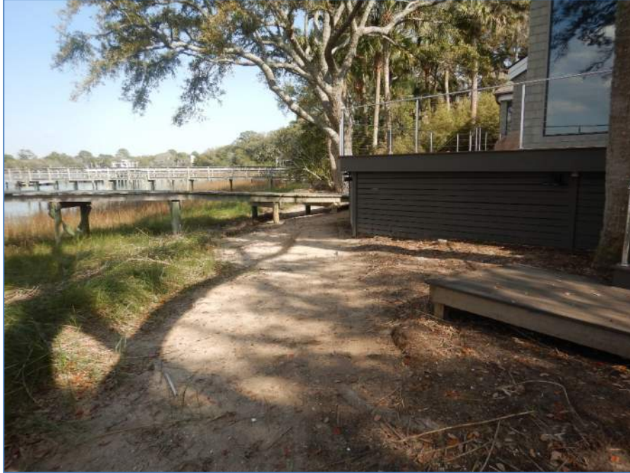
Photograph 3: Rear of Residence Rear Landing Out of Plumb
