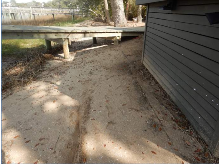
Photograph 5: Visible Impacts to Rear Deck
